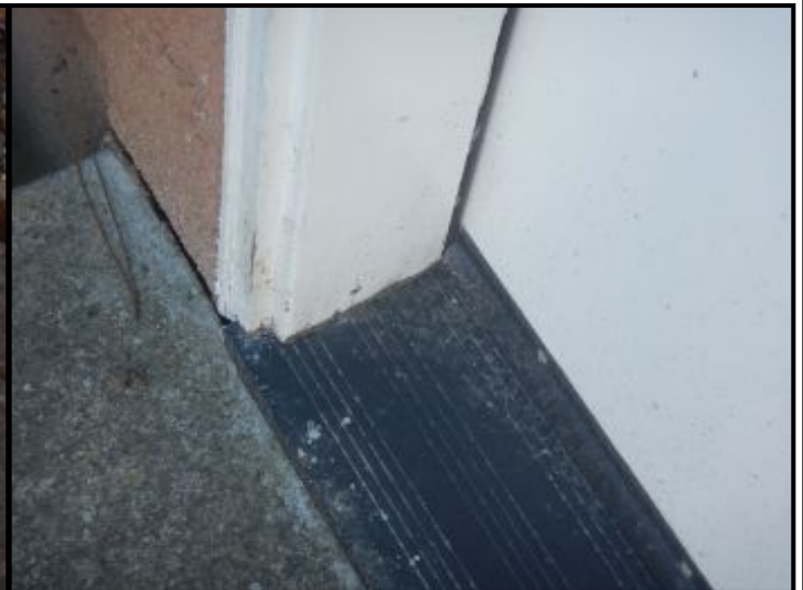
Door jamb damage to rear exterior door
