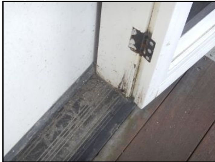
Door jamb damage at rear exterior door
