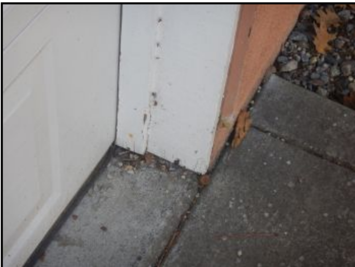
Trim damage at garage
