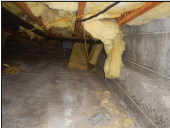
Fallen insulation in the sub area.
