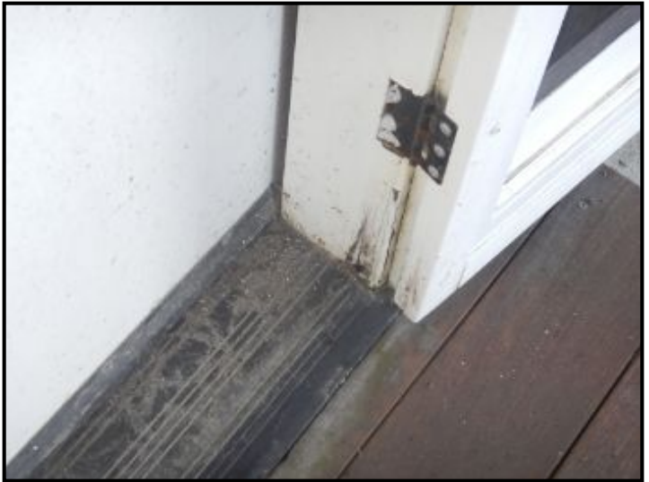
Door jamb damage at rear exterior door
