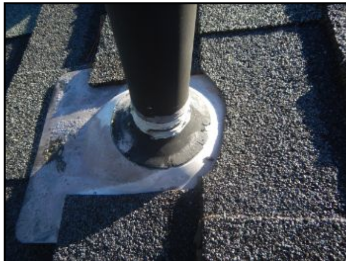
Worn storm collars at plumbing vents.
