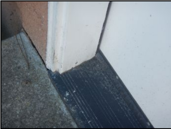
Door jamb damage to rear exterior door
