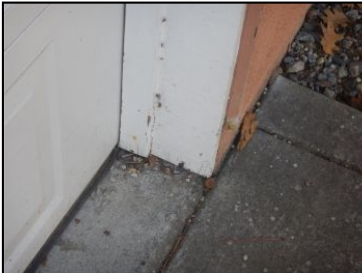
Trim damage at garage
