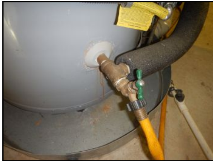
Encrustations at water heater
