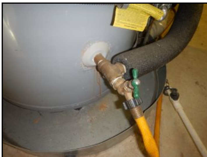
Encrustations at water heater
