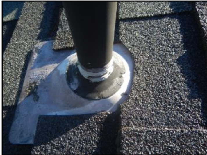
Worn storm collars at plumbing vents.
