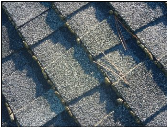
Moss growth at roof top.
