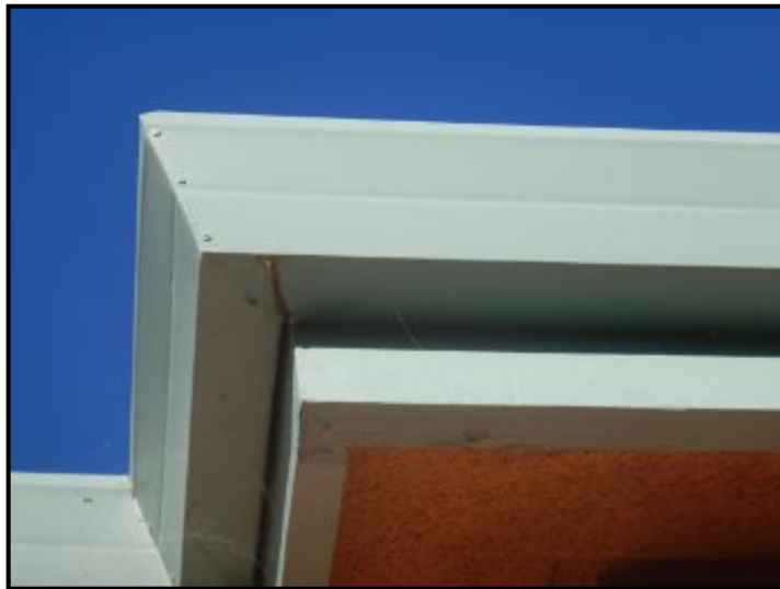
Leaking point at rear gutter seam.
