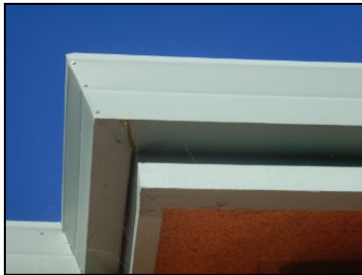
Leaking point at rear gutter seam.
