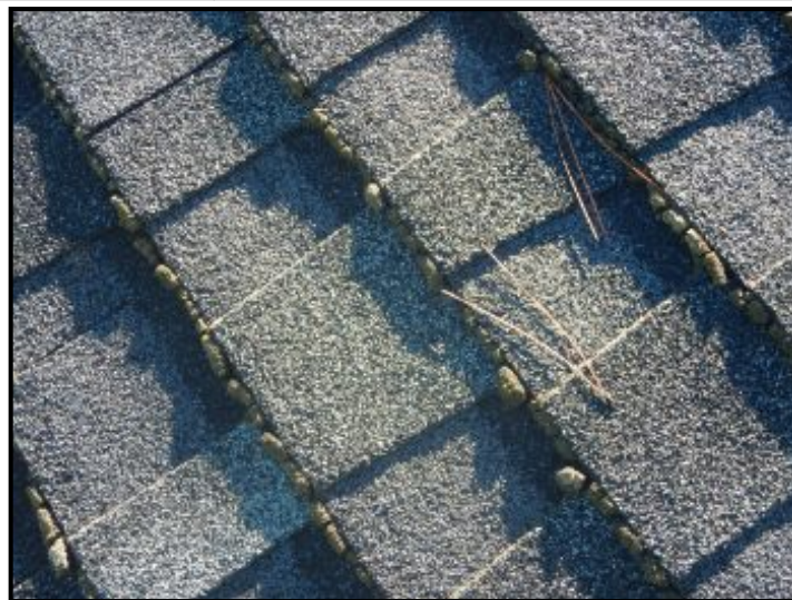
Moss growth at roof top.
