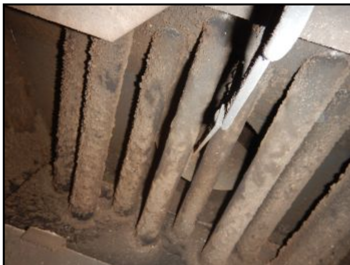
Soot build up at fireplace.
