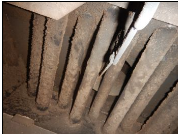
Soot build up at fireplace.
