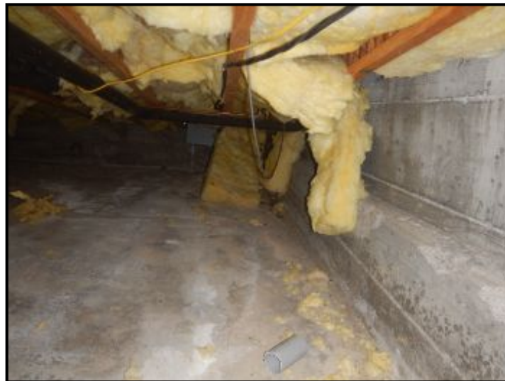
Fallen insulation in the sub area.
