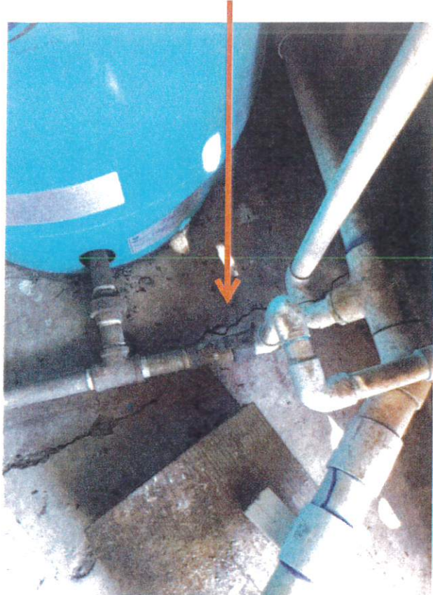
Domestic Pressure System Main Shut-off
