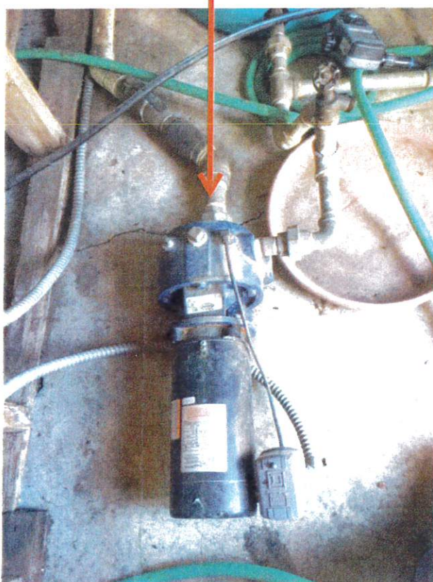
Domestic Booster Pump
