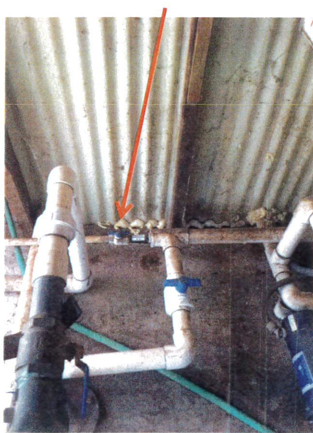
Guest House Shut-off
