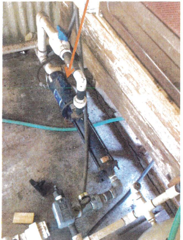
Vineyard Irrigation Booster Pump
