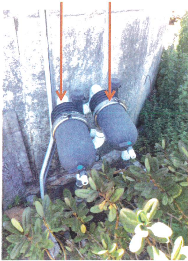
Lower Vineyard Irrigation Filters
