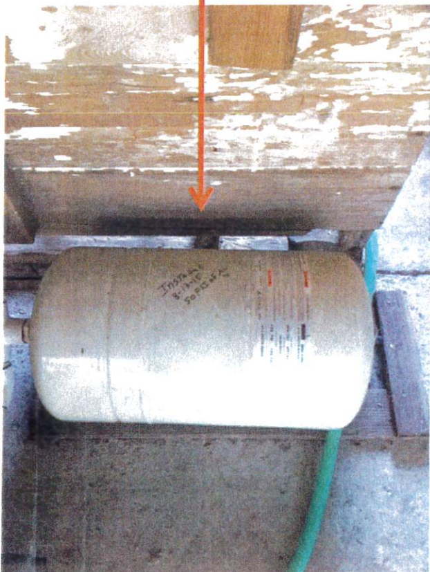
Vineyard Irrigation Expansion Tank
