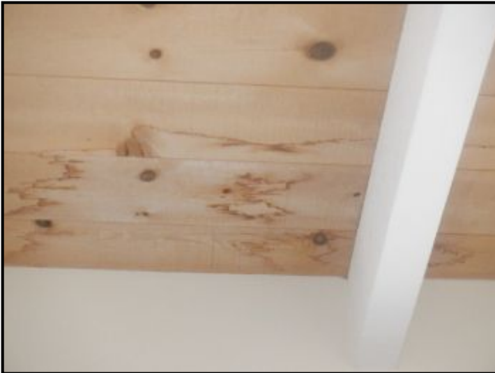
Moisture staining at dining room ceiling.
