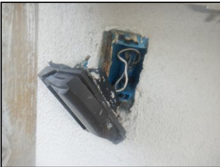
Loose electrical outlet in front of studio.
