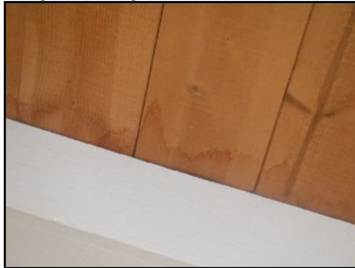
Moisture staining at ceiling.
