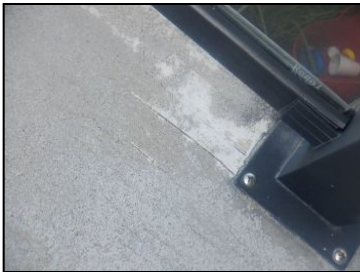
Worn surface at master bedroom deck.
