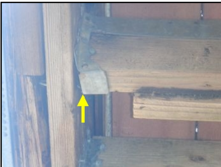
Joist hangers pulling away from deck fascia.
