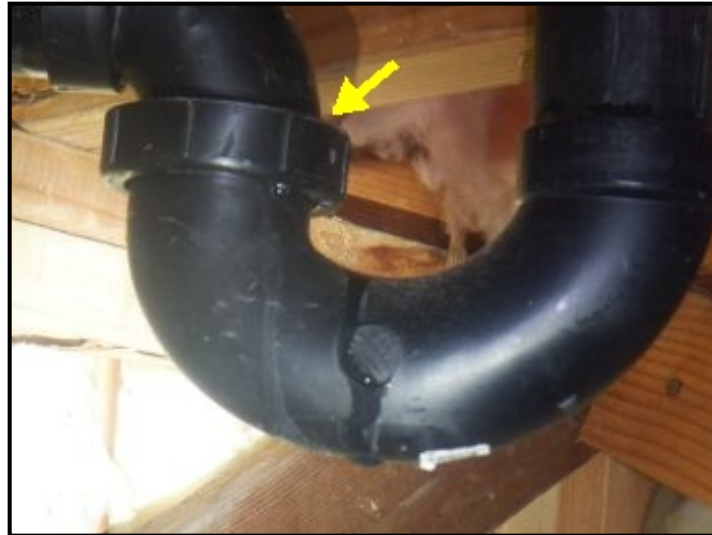
Leaking from shower drain line.
