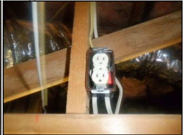
Missing cover plate in sub area.
