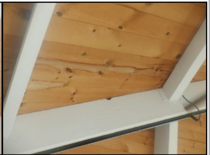
Moisture staining at loft ceiling.
