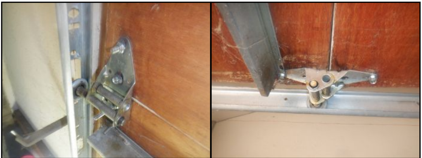
Loose roller brackets.
