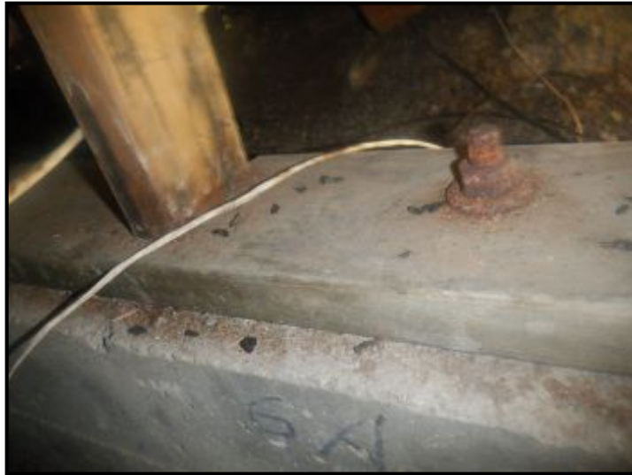
Rodent droppings in sub area.
