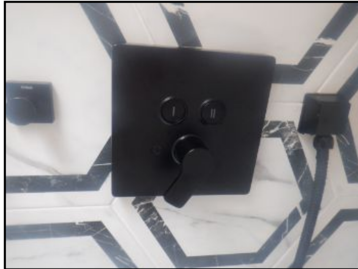
Loose shower fixture cover.
