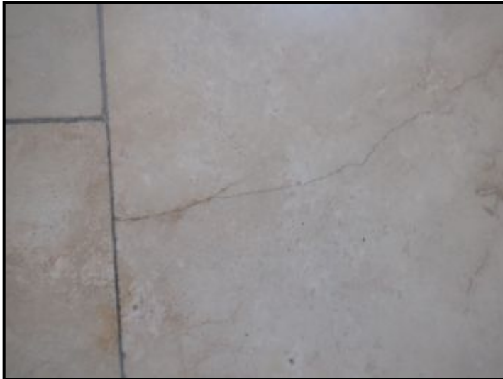
Cracked tiles at entry way.
