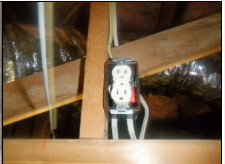
Missing cover plate in sub area.
