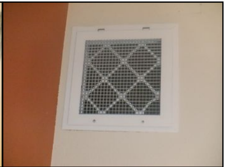
Replace air return filter.
