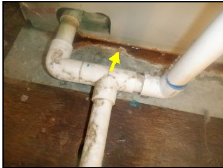
Leaking from furnace.
