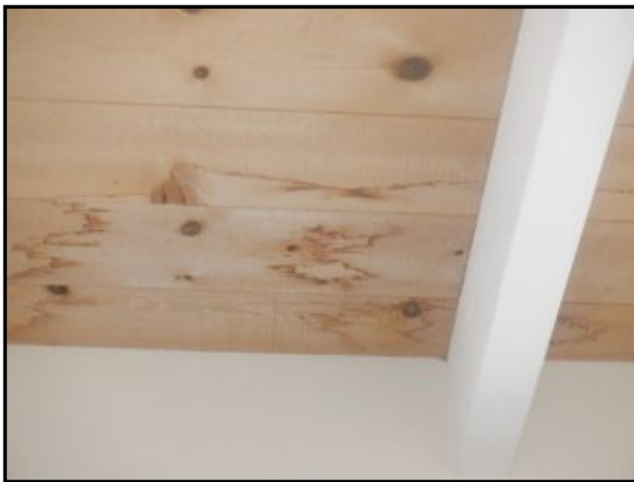
Moisture staining at dining room ceiling.
