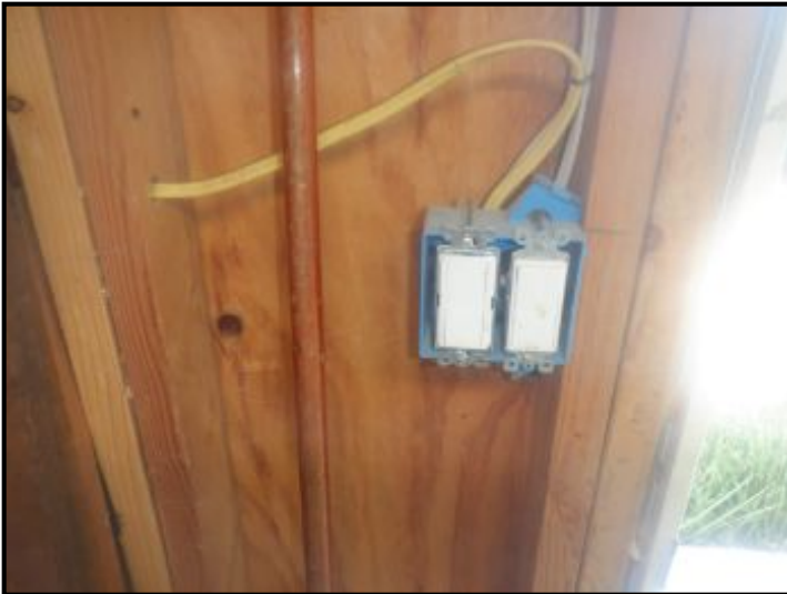
Missing cover plate in sub area.
