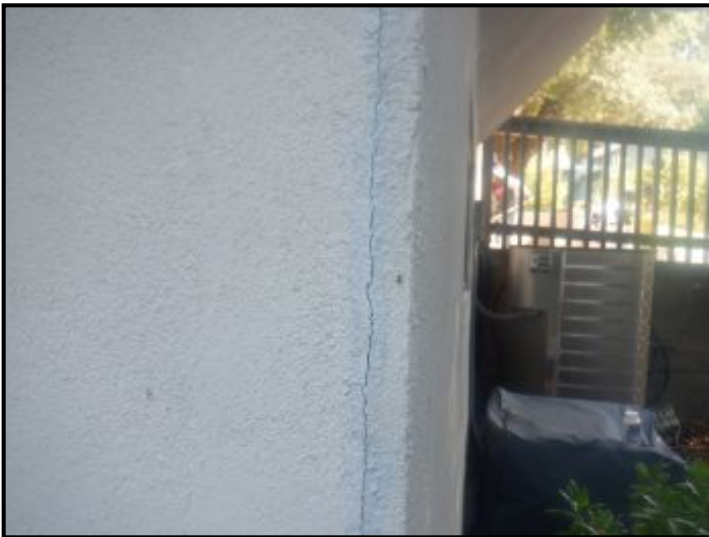
Seal stucco cracking as needed.
