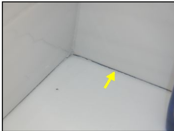
Grout voids around tub.
