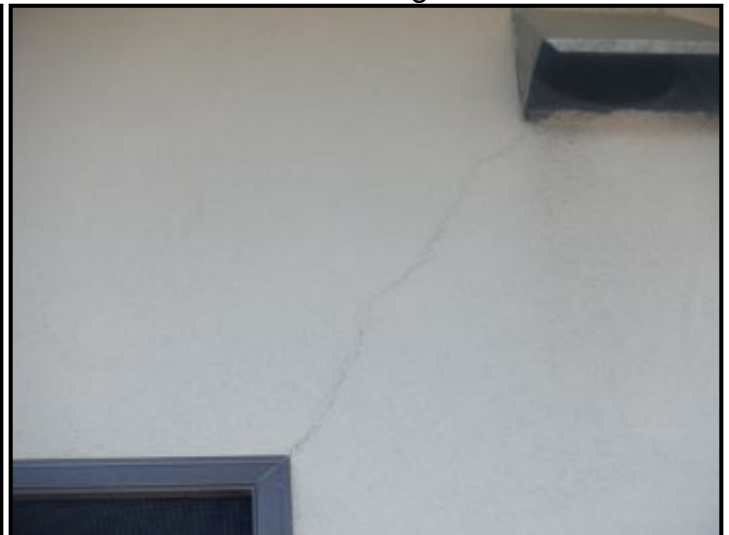
Seal stucco cracking as needed.
