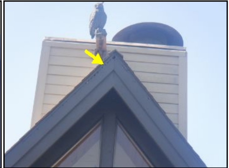
Bird damage at peak of roof.
