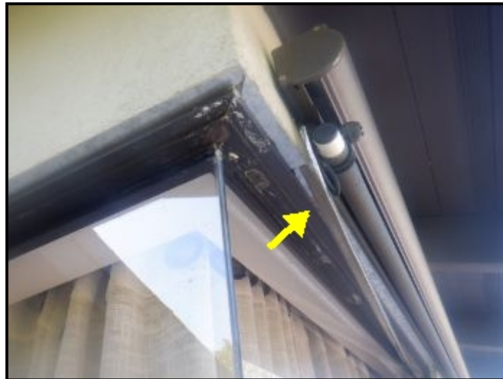
Loose weather stripping around window.
