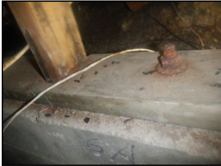
Rodent droppings in sub area.
