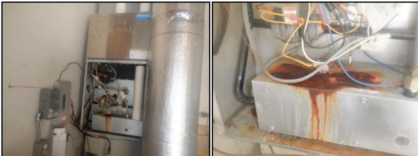
Staining at interior of furnace
