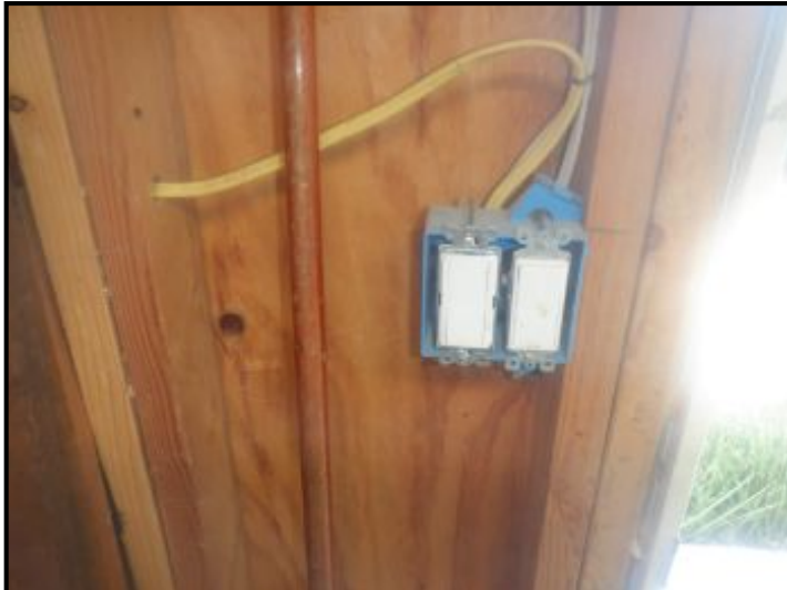
Missing cover plate in sub area.
