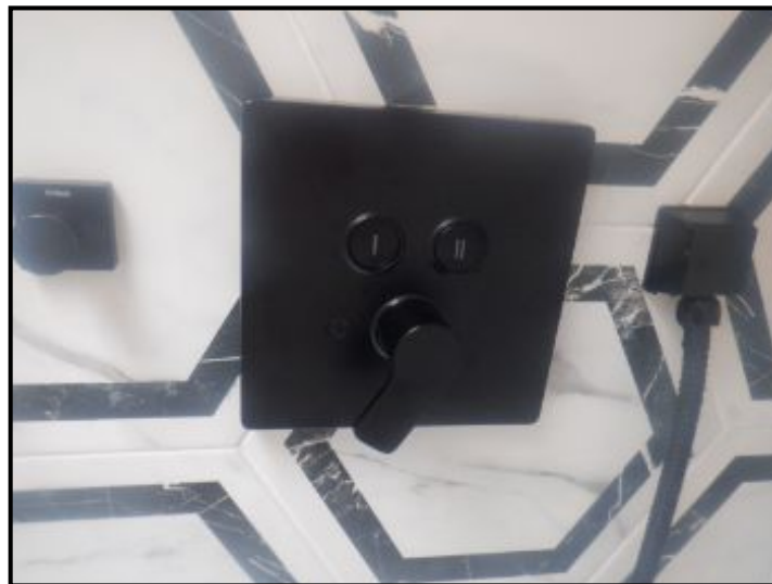
Loose shower fixture cover.
