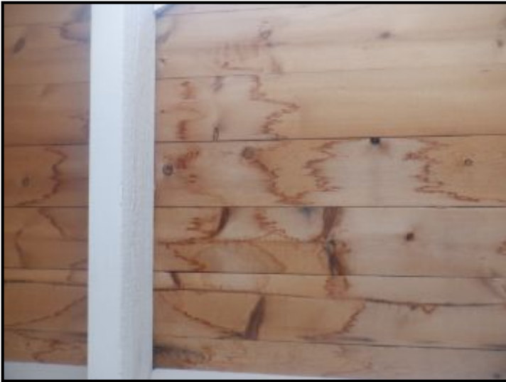
Moisture staining below skylight.
