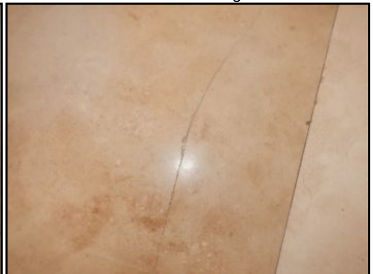
Cracked tiles at entry area.
