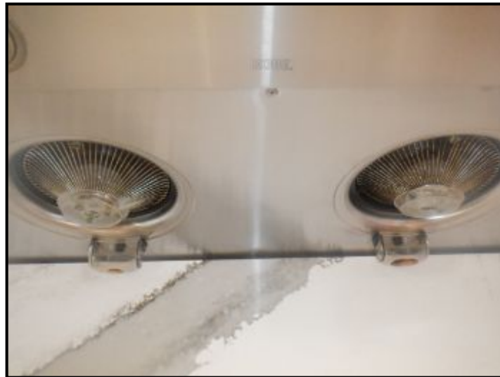
Grease build up at stove top exhaust.
