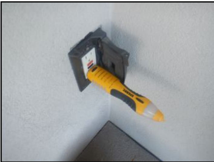
Deck GFCI not resetting.
