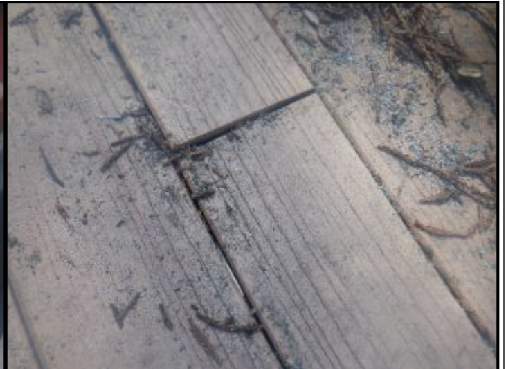
Lifted deck board.
