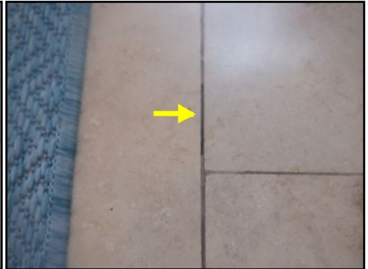
Grout voids at dining area.
