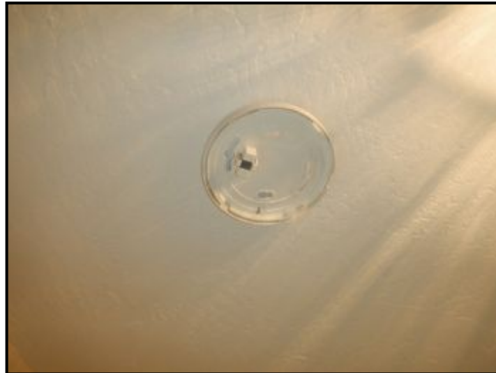
Missing smoke detector.
