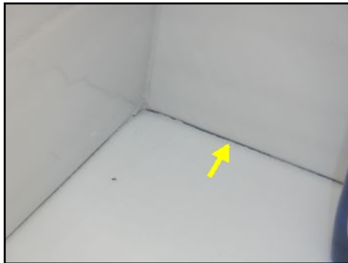
Grout voids around tub.
