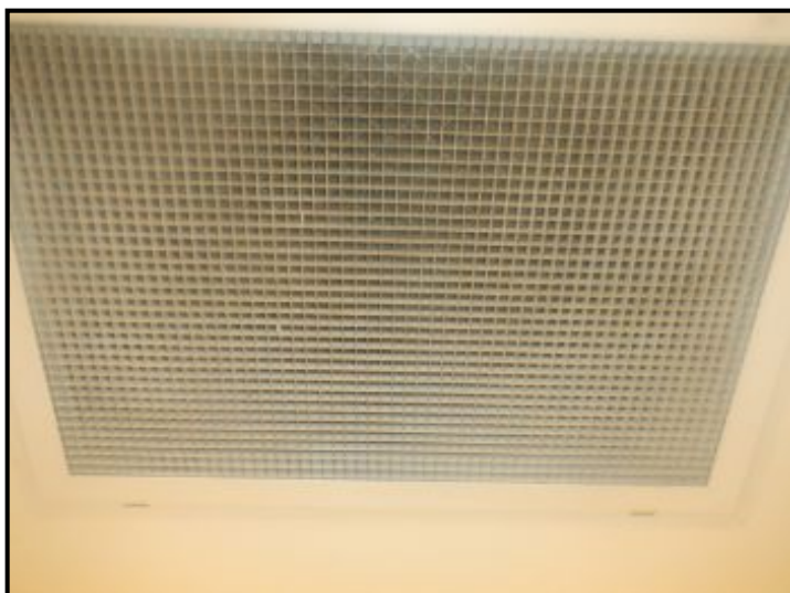
Replace air return filters.
