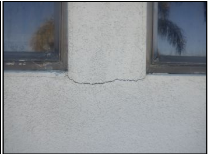
Seal stucco cracking as needed.
