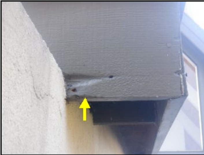
Fascia damage at right side of home.
