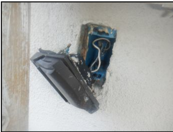
Loose electrical outlet in front of studio.
