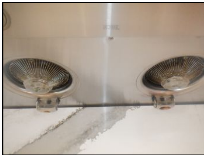
Grease build up at stove top exhaust.
