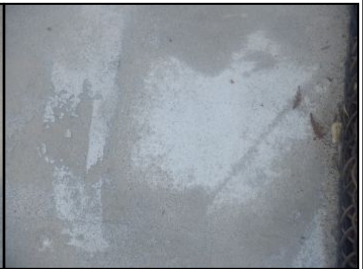
Worn surface at master bedroom deck.
