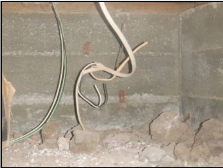
Exposed electrical in sub area.
