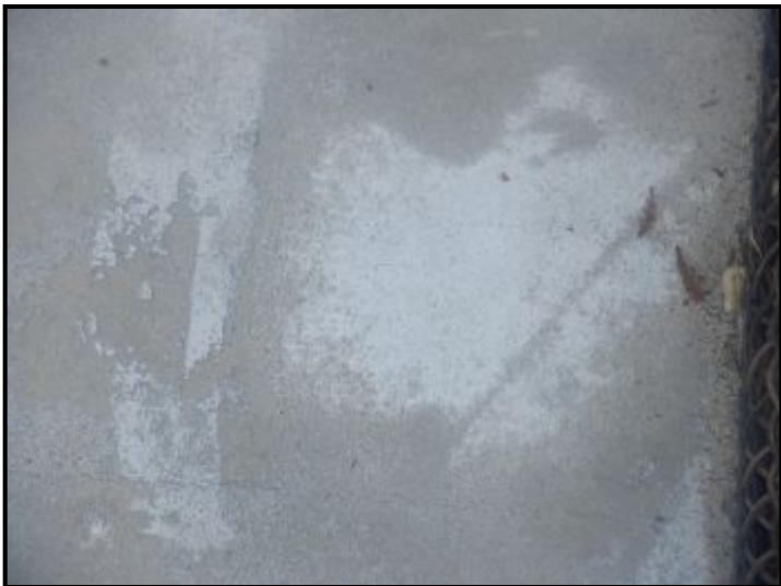
Worn surface at master bedroom deck.
