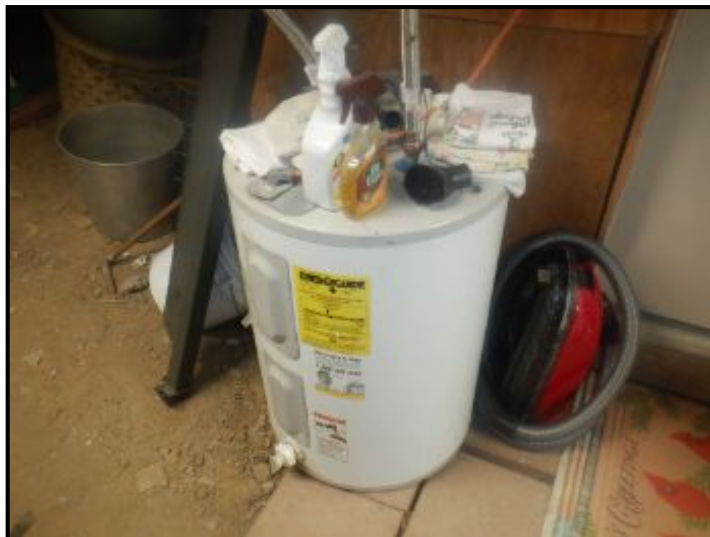
Water heater not properly strapped.
