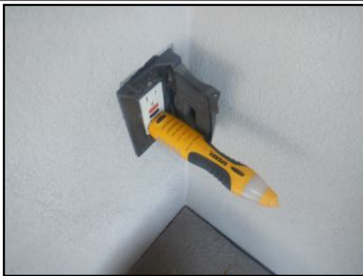
Deck GFCI not resetting.
