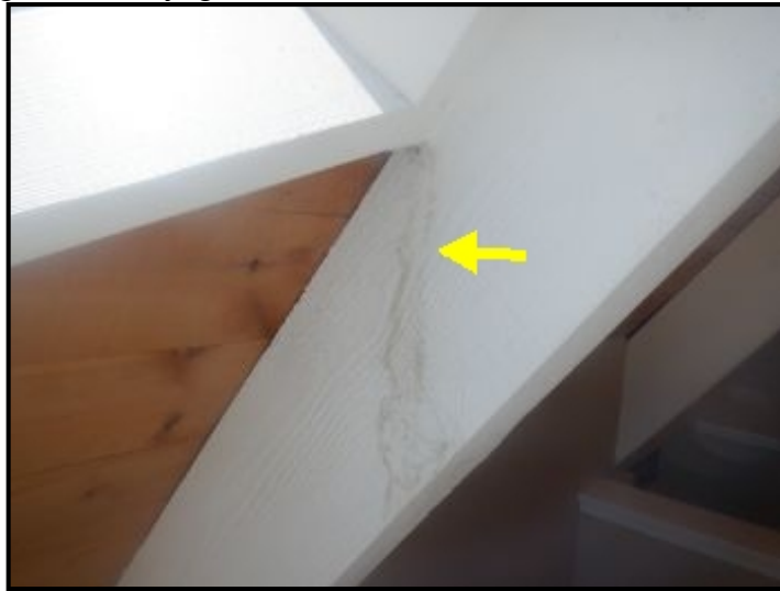
Moisture staining at skylight.
