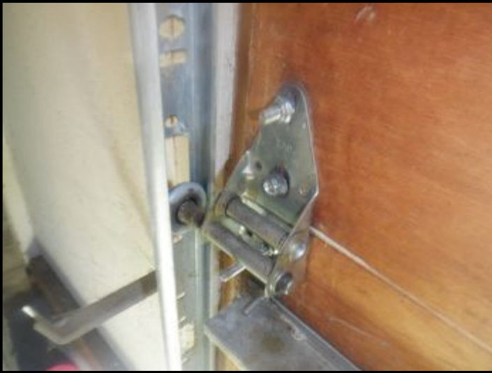
Loose roller brackets.
