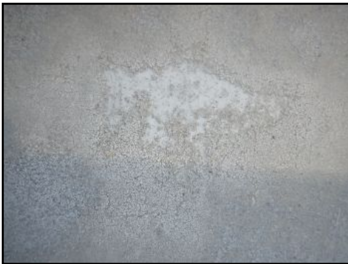
Worn surface at master bedroom deck.
