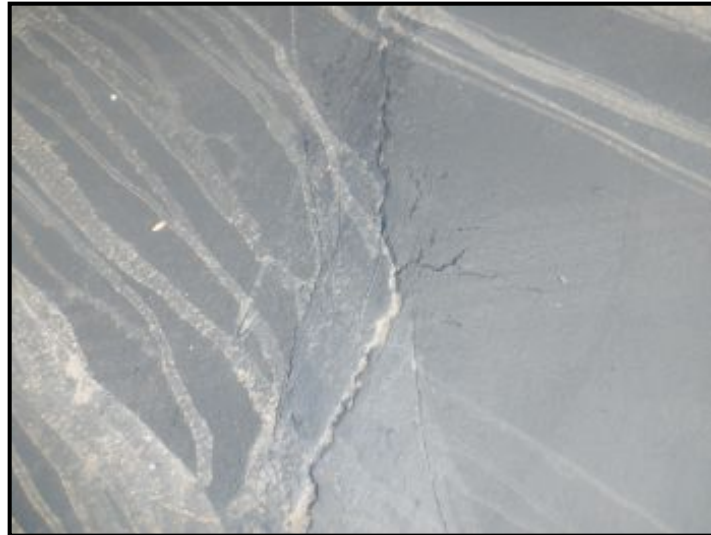
Cracking at driveway
