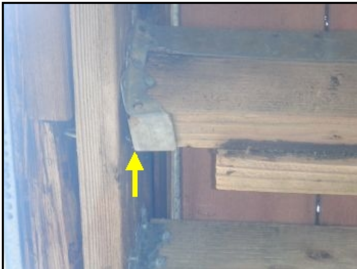
Joist hangers pulling away from deck fascia.
