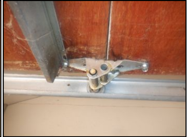
Loose roller brackets.
