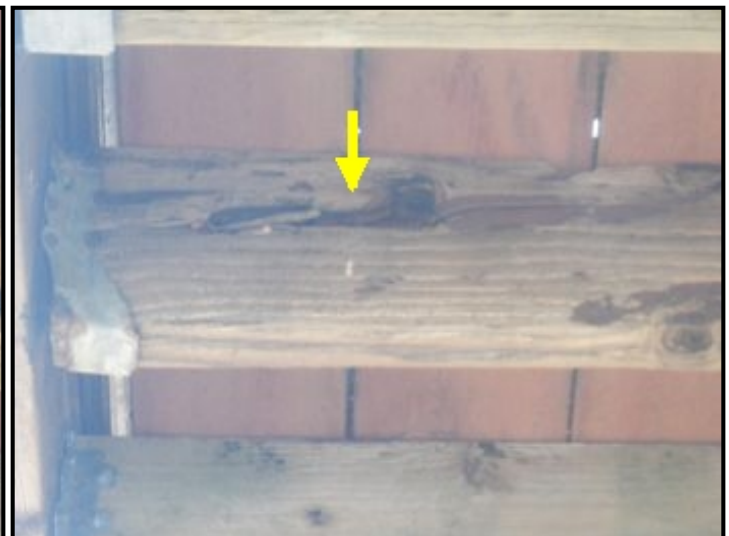
Damage to deck joist.
