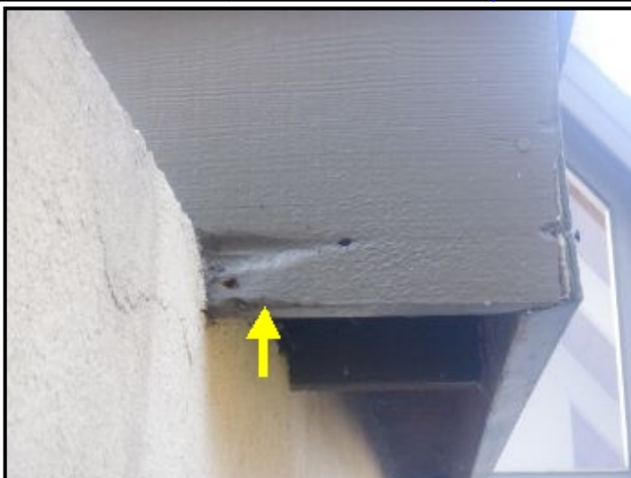
Fascia damage at right side of home.
