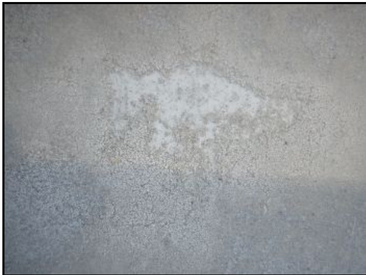
Worn surface at master bedroom deck.
