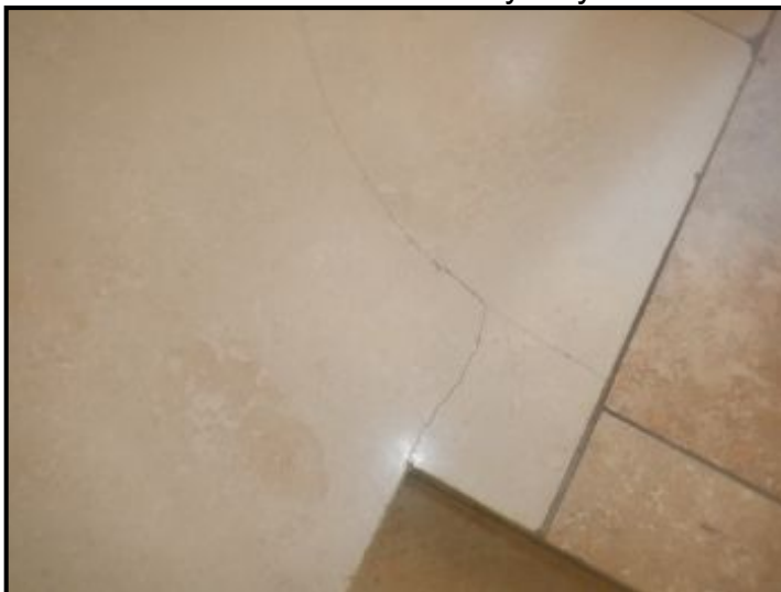
Cracked tiles at entry area.
