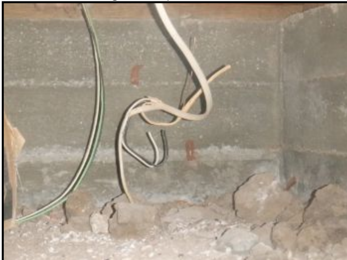
Exposed electrical in sub area.
