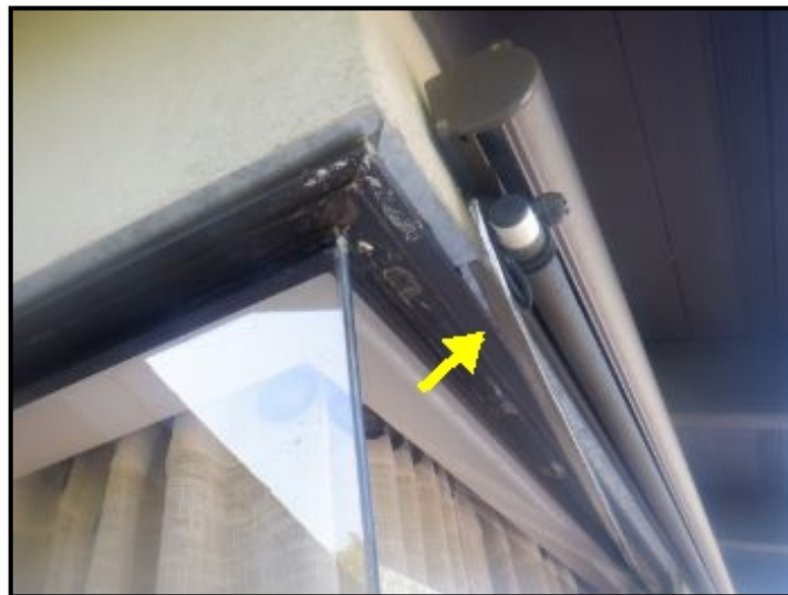
Loose weather stripping around window.
