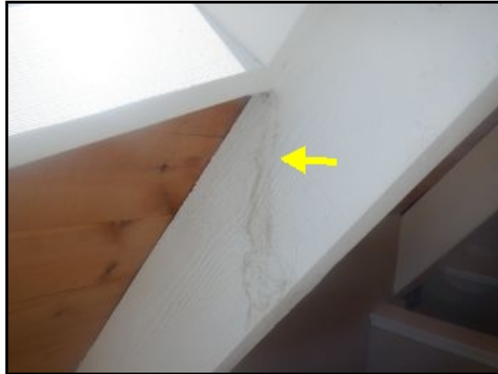
Moisture staining at skylight.
