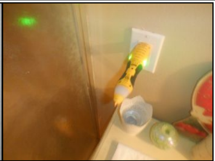
Outlet next to studio shower not GFCI
