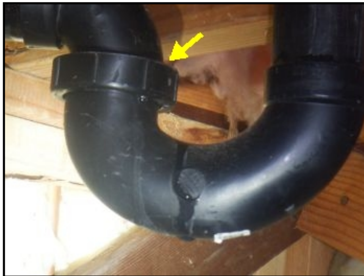
Leaking from shower drain line.
