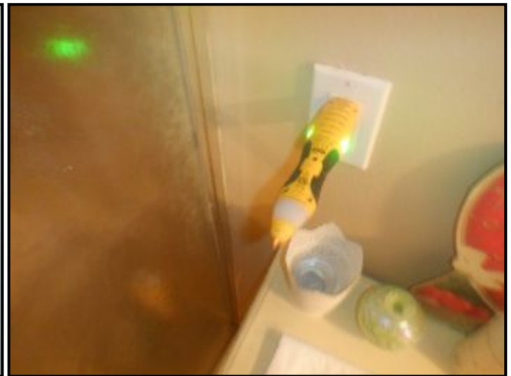
Outlet next to studio shower not GFCI
