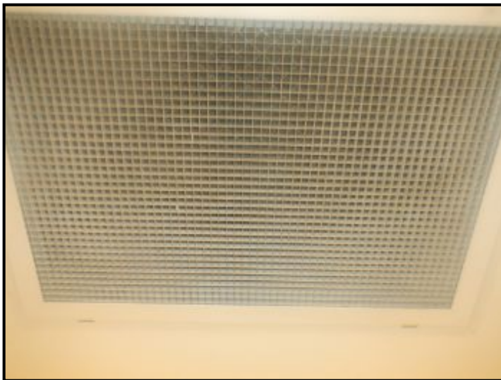
Replace air return filters.
