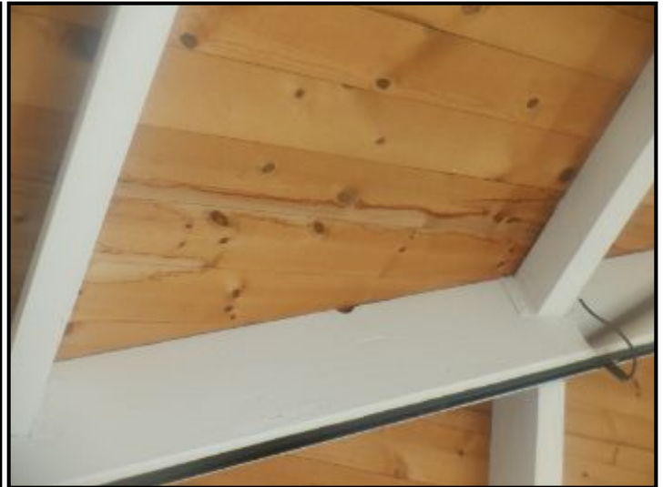
Moisture staining at loft ceiling.
