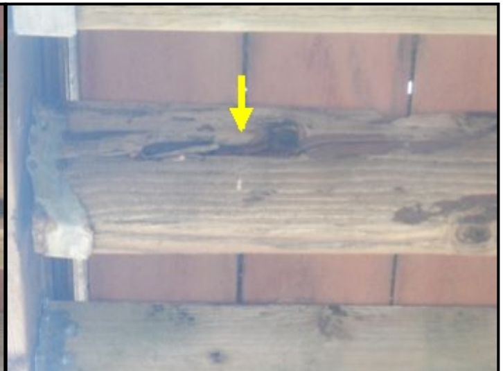
Damage to deck joist.
