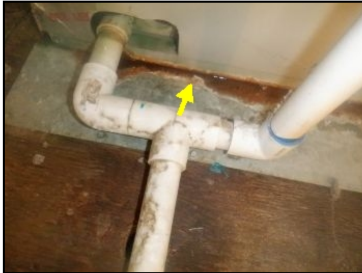
Leaking from furnace.
