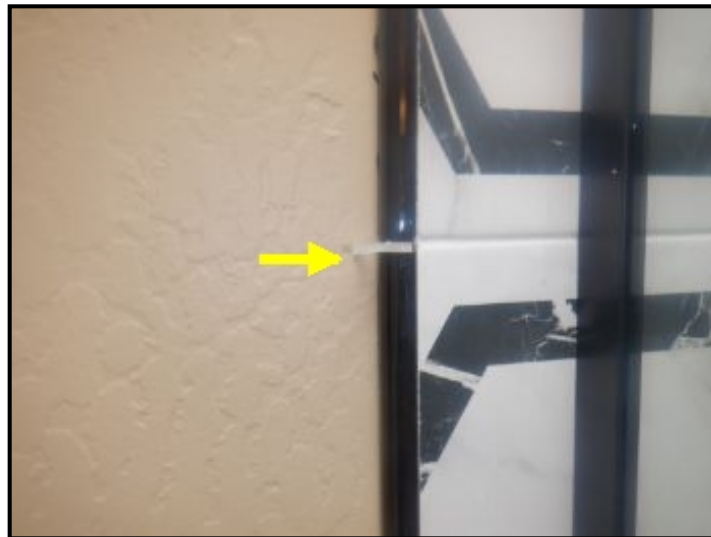
Grout voids around tiles.
