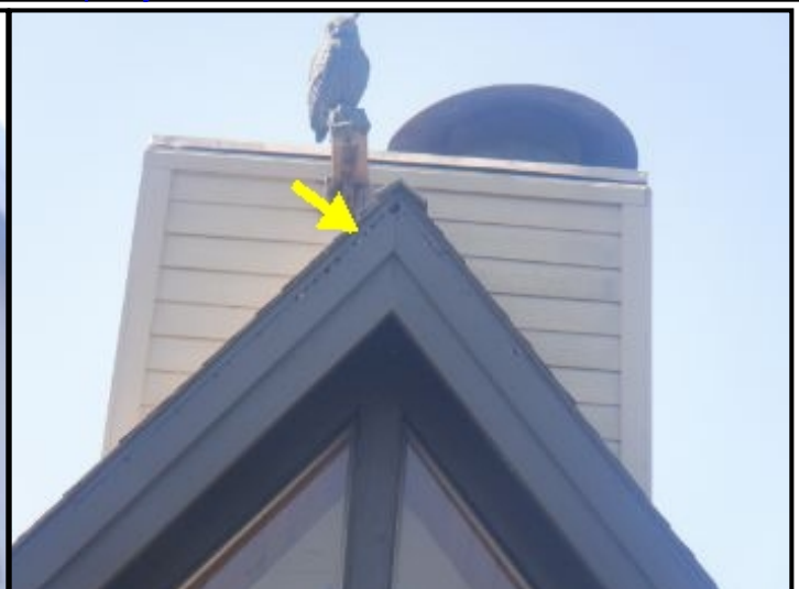
Bird damage at peak of roof.
