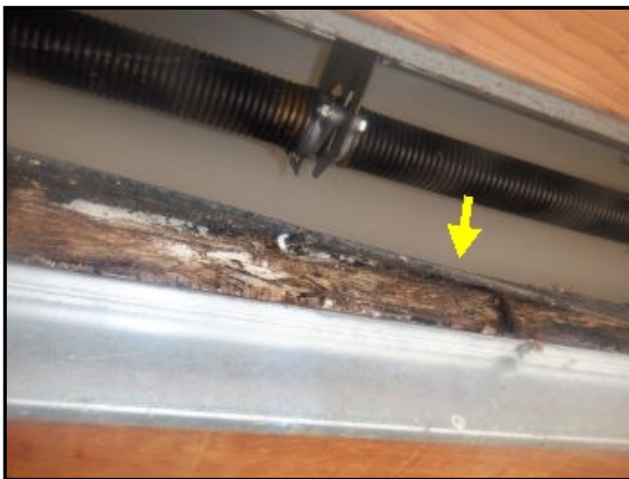
Deteriorated garage door seal.
