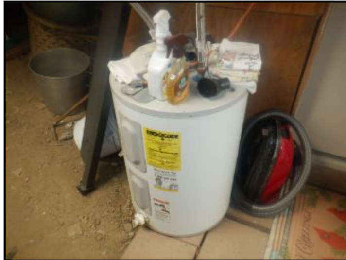
Water heater not properly strapped.
