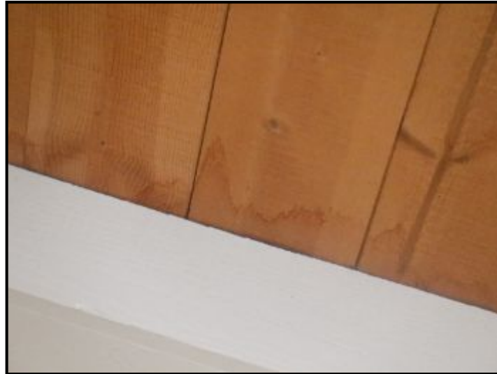
Moisture staining at ceiling.
