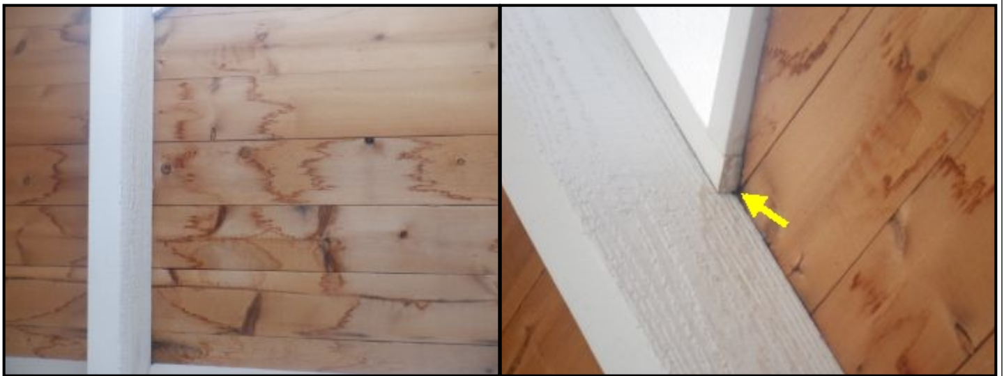
Moisture staining below skylight.
