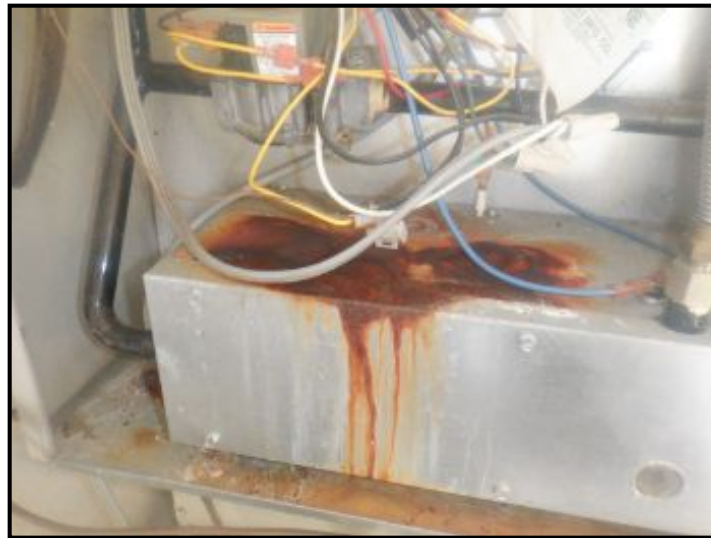
Staining at interior of furnace
