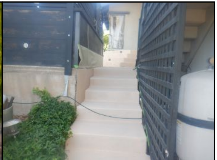
No handrail installed at stairway.
