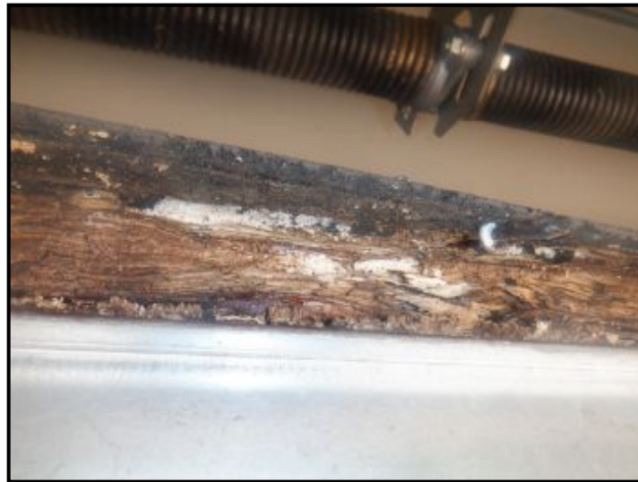
Wood damage to bottom panel of garage door.
