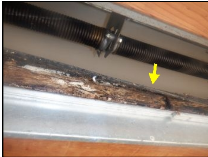
Deteriorated garage door seal.
