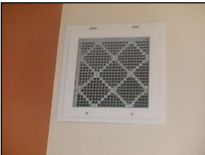
Replace air return filter.
