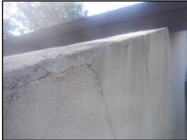
Seal stucco cracking as needed.
