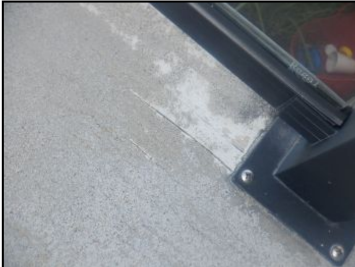
Worn surface at master bedroom deck.
