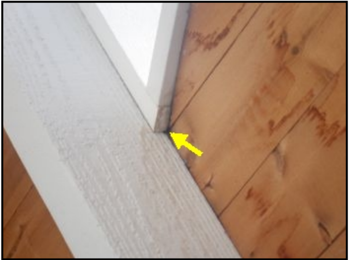
Moisture staining at skylight.
