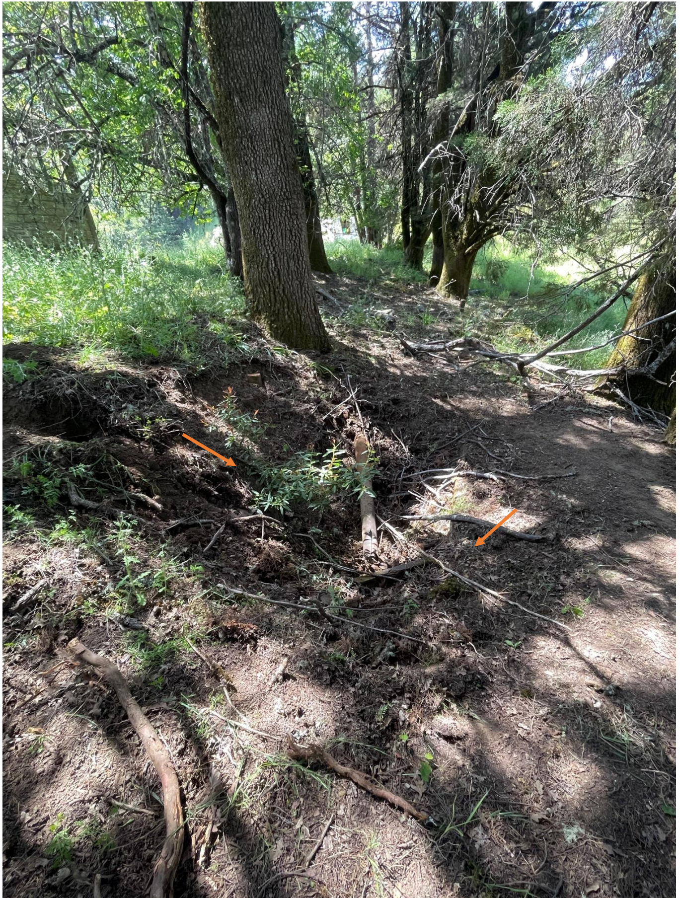
Location of the collapsed cesspool
