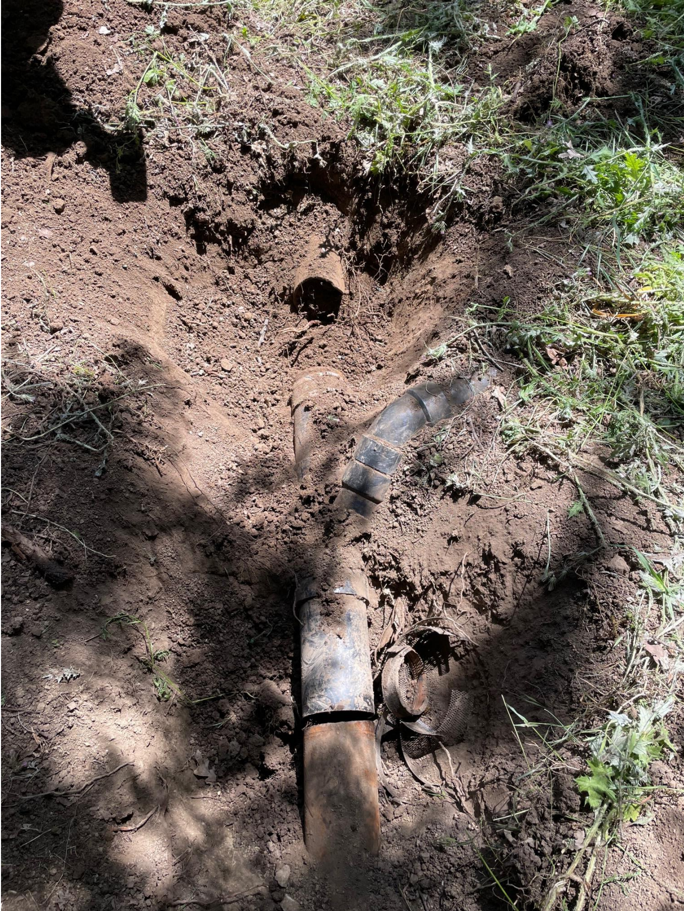
Solid sewer line from house to the cesspool
