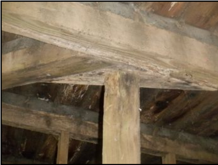
Damage to under side of deck.
