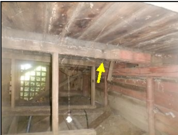
Sagging support beam under deck.
