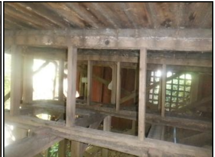
Sub standard and damaged supports under deck.
