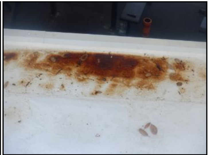
Indications of past standing water at roof top.
