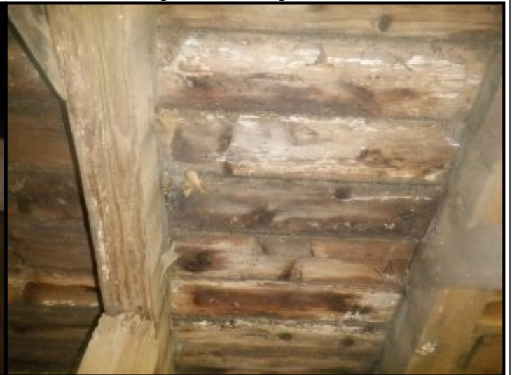
Fungus to under side of deck.
