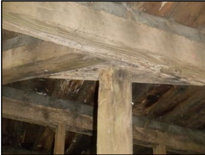
Damage to under side of deck.
