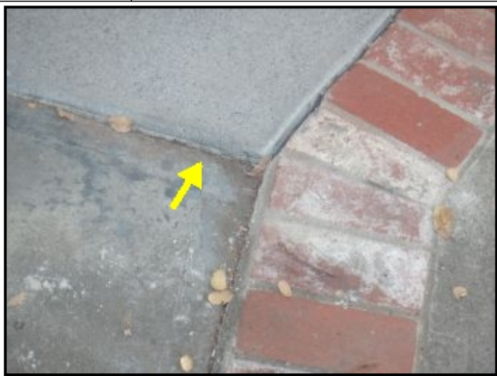
Uneven concrete walkway at front of home.
