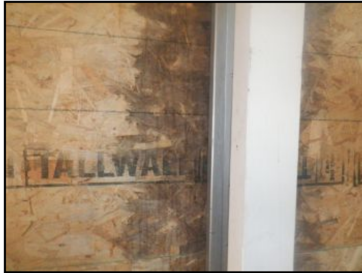
Moisture staining to garage door.
