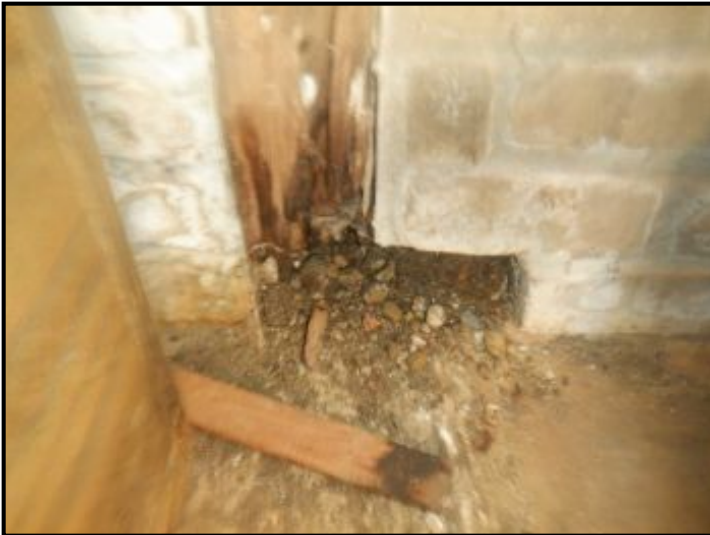
Post damage at brick foundation.
