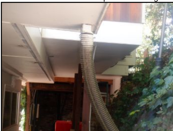
Loose drain pipe used at downspout.
