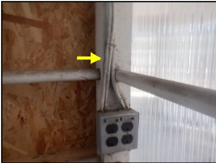
Unprotected Romex in garage area.
