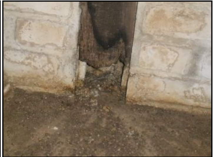
Post damage at brick walls.
