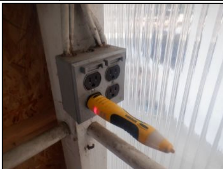
Ungrounded outlets in garage.
