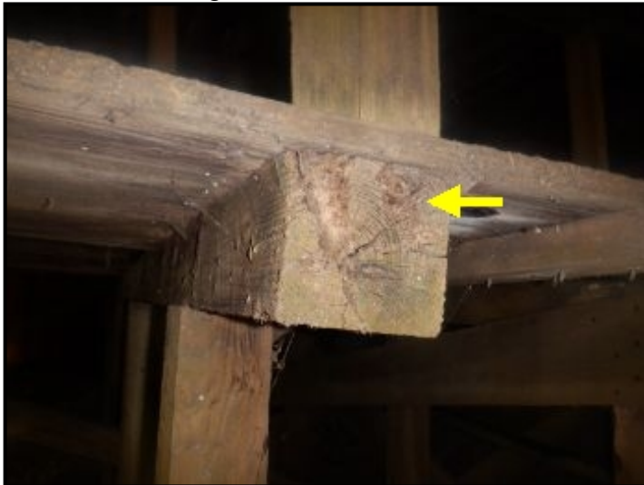
Damage to framing under deck.
