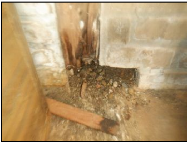
Post damage at brick foundation.
