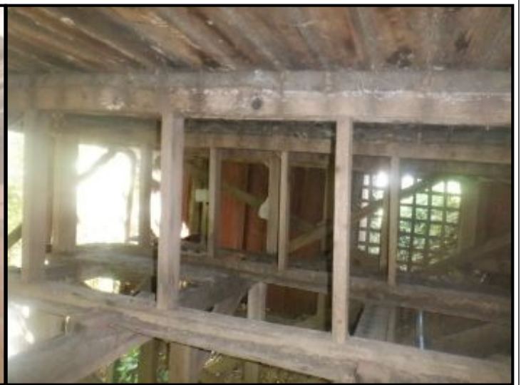
Sub standard and damaged supports under deck.
