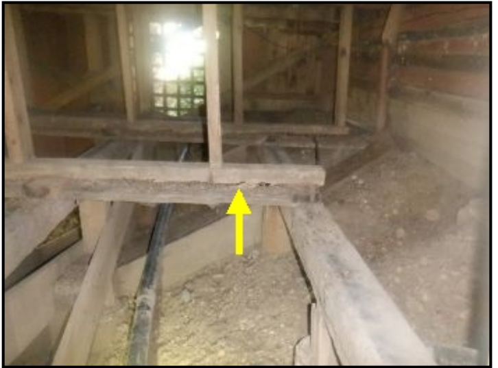
Damage to framing under deck.
