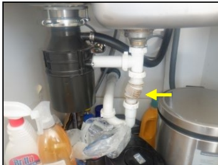
Flex drain line installed in granny unit.
