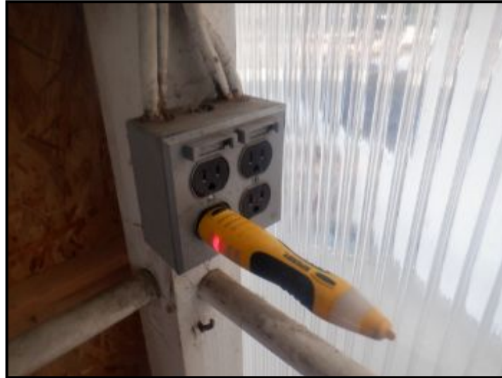
Ungrounded outlets in garage.
