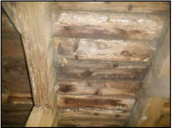
Fungus to under side of deck.
