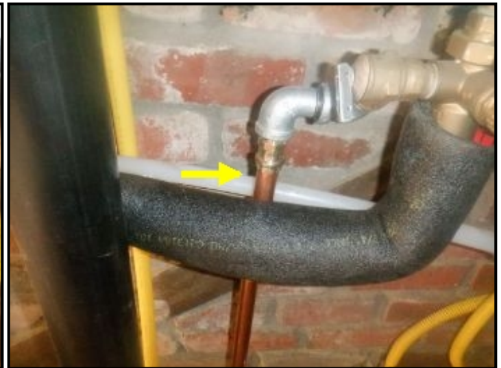
Discharge pipe installed at water heater.
