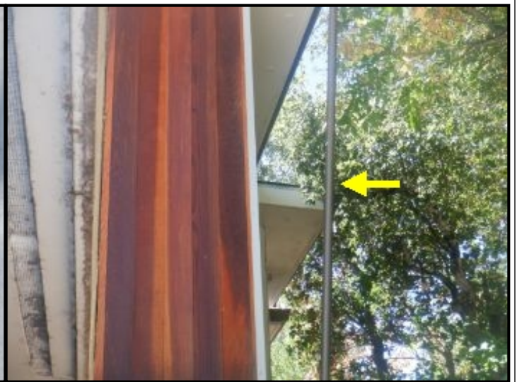
Downspout not secured to structure.
