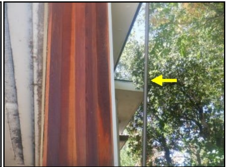
Downspout not secured to structure.
