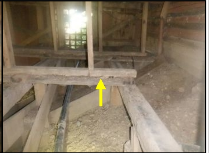
Damage to framing under deck.
