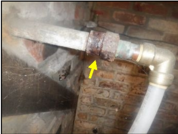
Leaking at supply line under granny unit.
