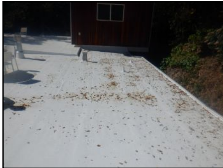
Debris on roof.
