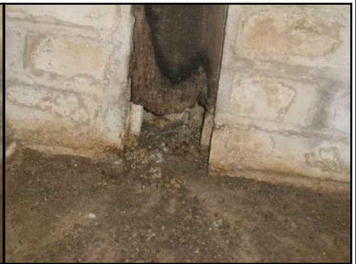
Post damage at brick walls.
