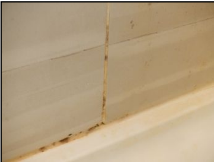
Mildew at granny unit shower caulking.
