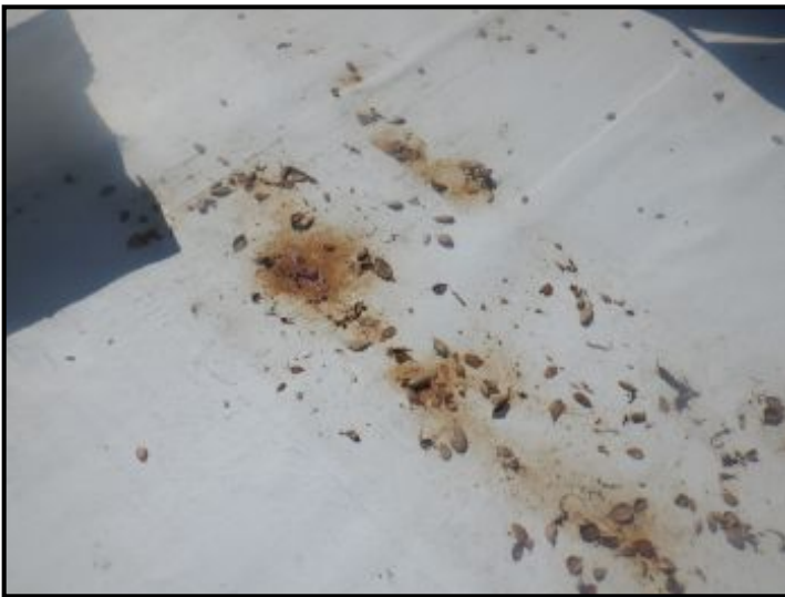
Staining indicating past standing water.
