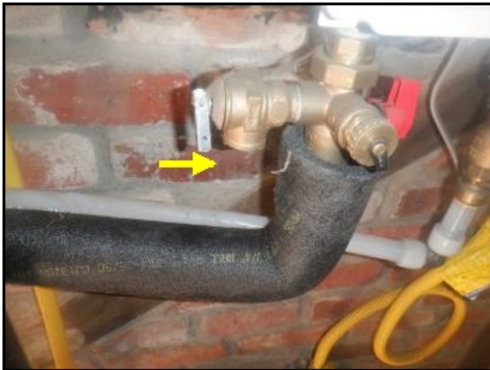
Missing drain pipe at water heater TPR valve.
