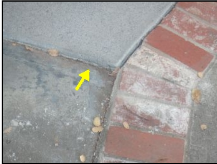
Uneven concrete walkway at front of home.
