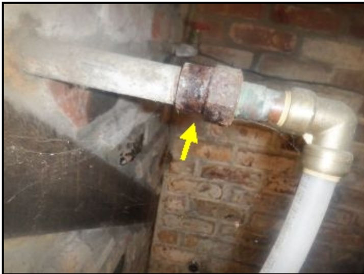
Leaking at supply line under granny unit.
