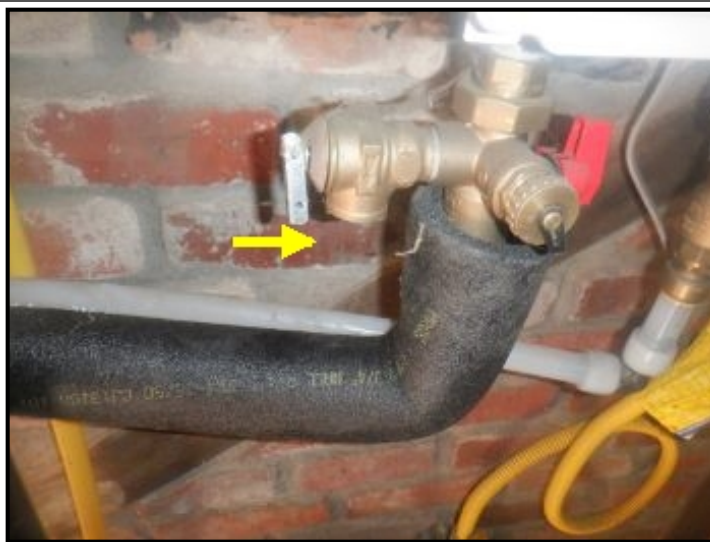
Missing drain pipe at water heater TPR valve.
