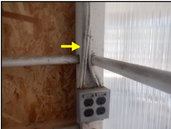
Unprotected Romex in garage area.
