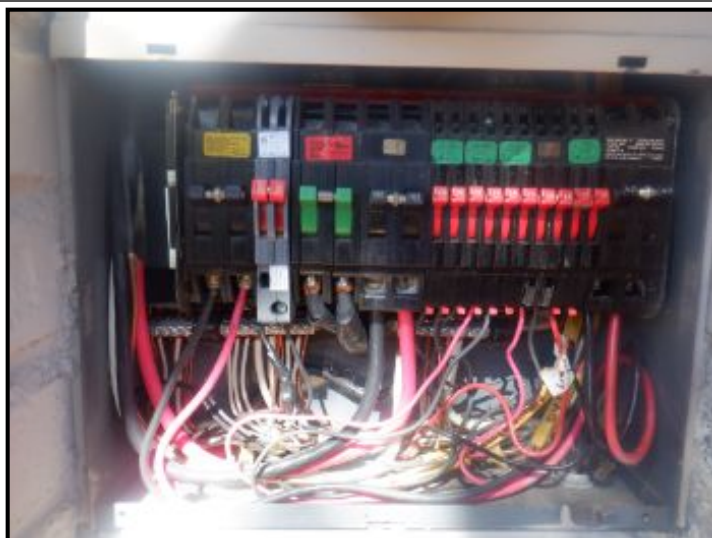
Zinsco panel installed at home.
