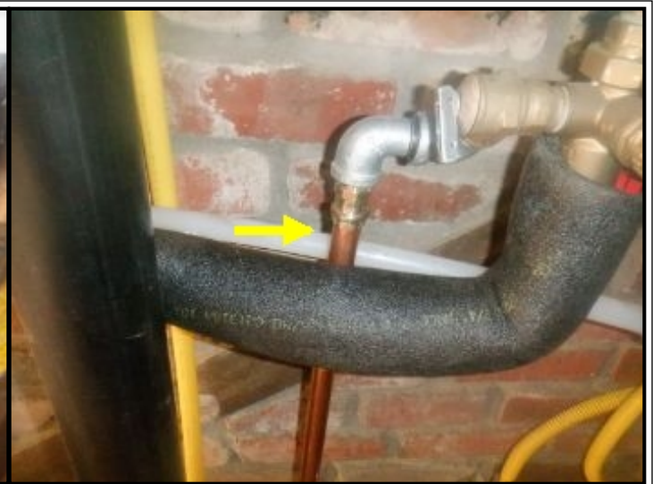
Discharge pipe installed at water heater.
