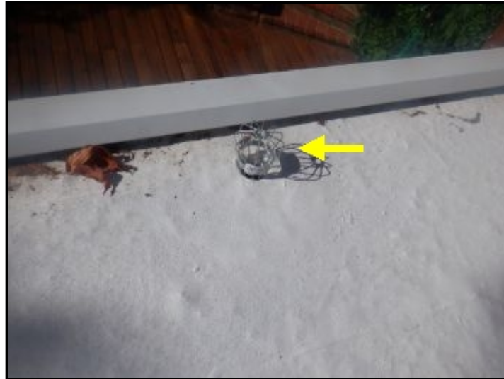
Screens installed at roof top drains.
