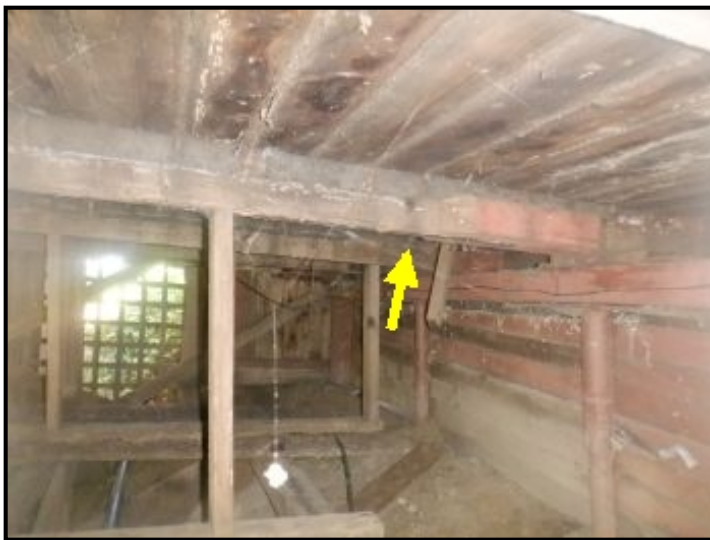
Sagging support beam under deck.
