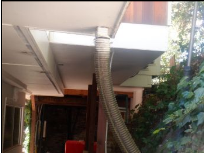
Loose drain pipe used at downspout.
