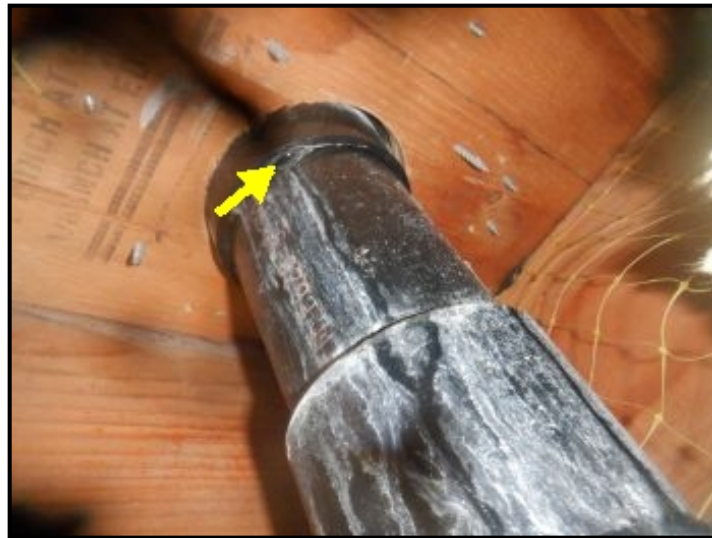
Leaking from toilet drain line.
