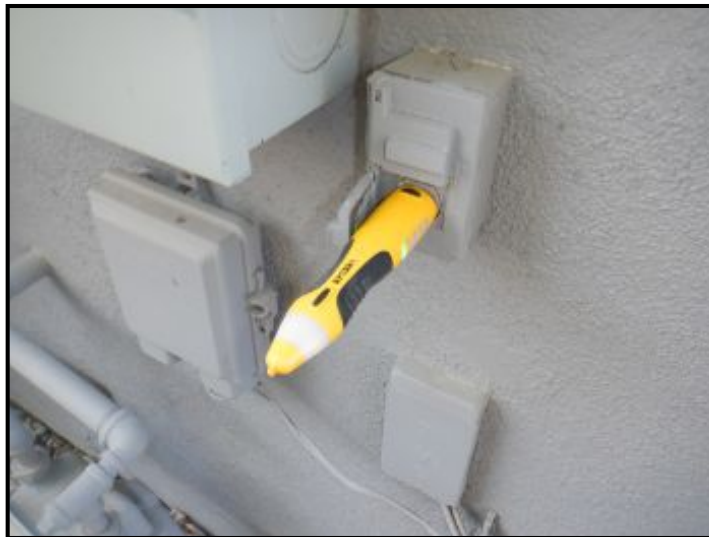
Exterior outlets are not GFCI protected.
