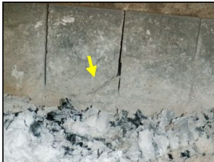
Cracked bricks at interior of fireplace.
