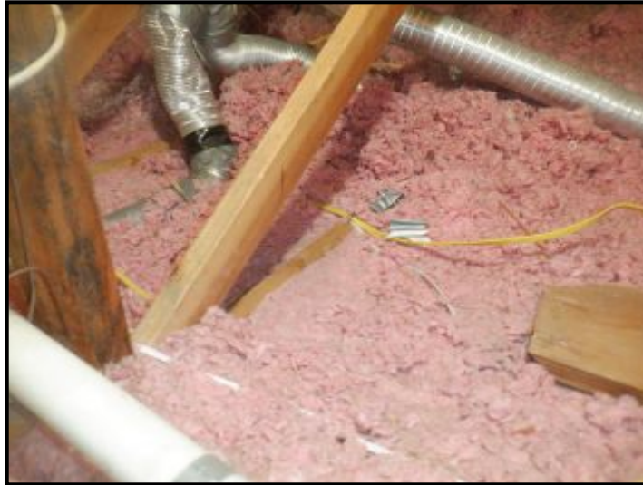
Low levels of insulation in attic.
