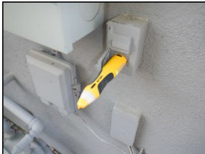
Exterior outlets are not GFCI protected.
