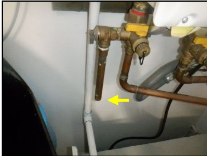
Discharge line does not terminate to the ground.
