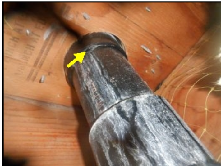
Leaking from toilet drain line.
