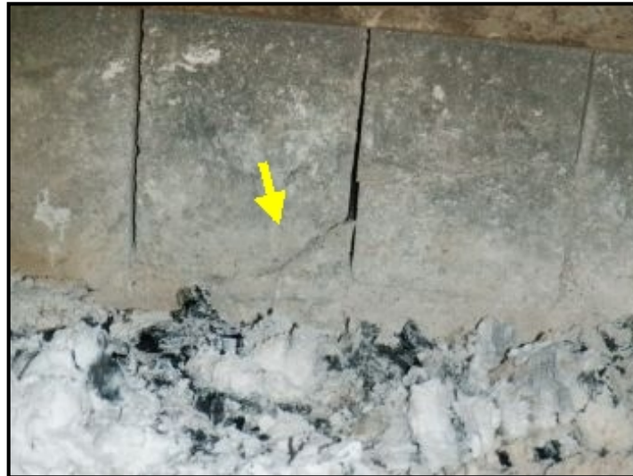
Cracked bricks at interior of fireplace.
